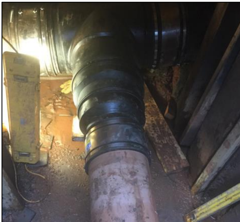
Figure 2: Temporary connection to existing 300m diameter sewer (at the top of the picture) in Station Road.
